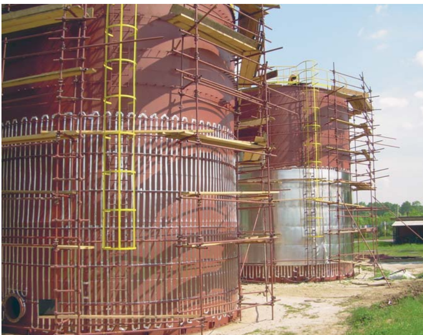
Heating cables assembled on tanks
